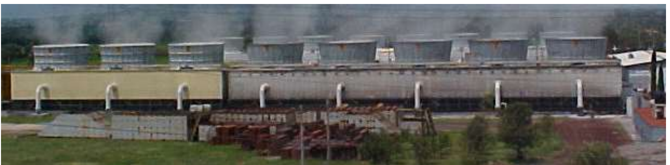
Conventional power plant cooling tower, comprising of 8 cells
